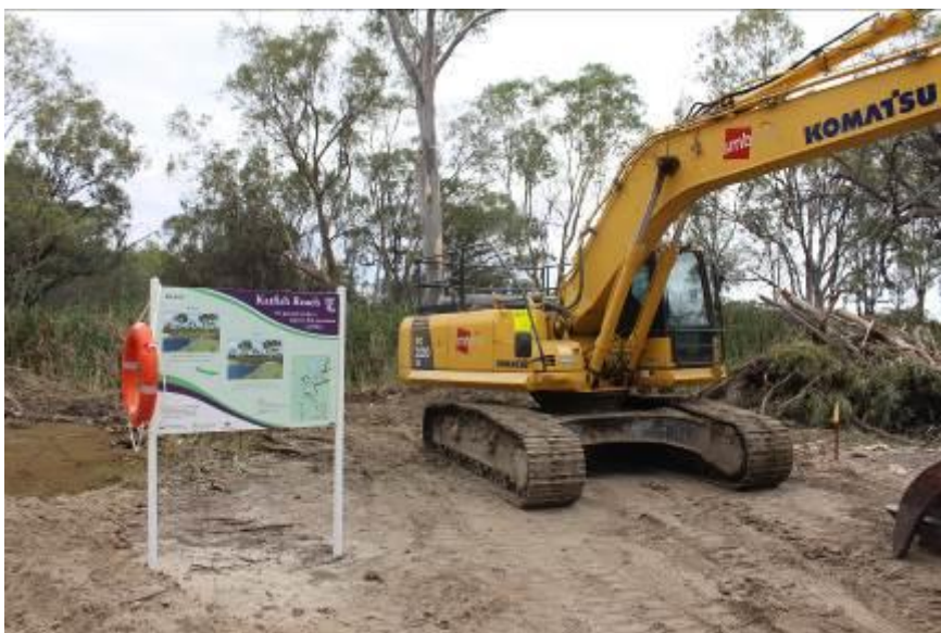
Photo 1: Excavation equipment onsite at Katfish Reach for the start of construction of a package of surface water management infrastructure.
